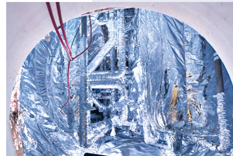
Segment of the cryogenic system that cools the LHC's superconducting magnet
