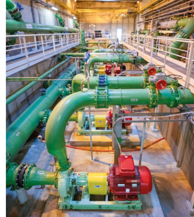
CERN's cooling and ventilation system equipped with ABB smart sensors
